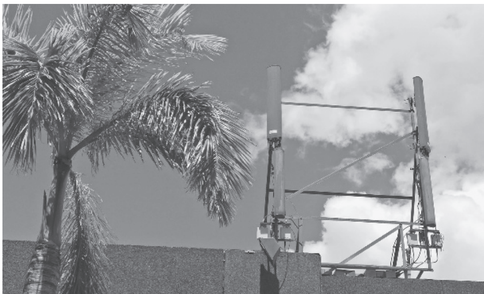
FIGURE 10-9 Cellsite with Paddle Antennas
